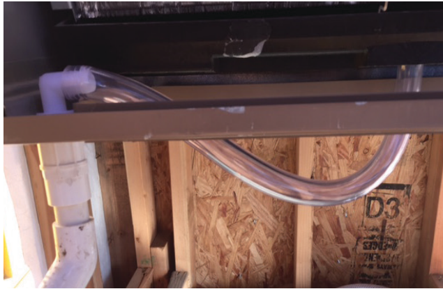
Figure 32: Inside of unit at return-air duct flange, showing sealed condensate tube opening
