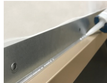
Figure 16: Caulk seal outside joints of wall sleeve before inserting into wall opening.
